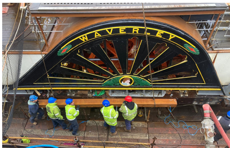
With the beam in place new belting was then installed before new steel facing bar was attached.
