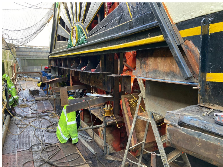
With the old beam removed the steel work within the support brackets could be addressed.
