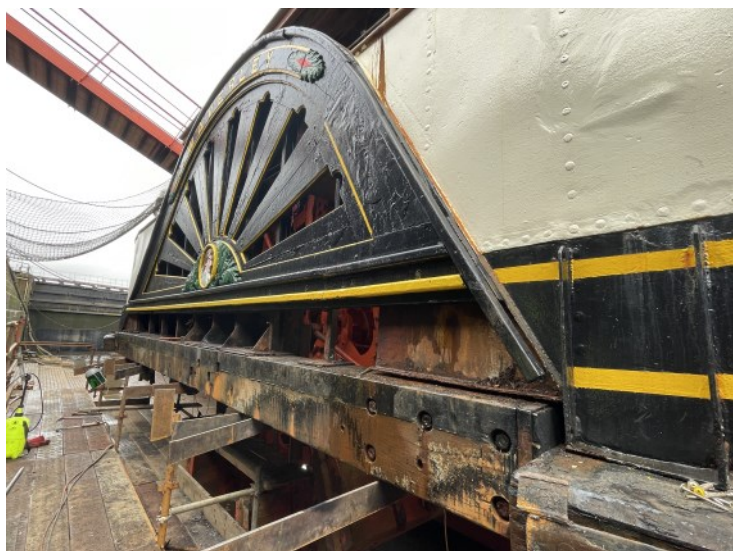
Step 1 was to remove the belting to gain access to the old spring beam.
